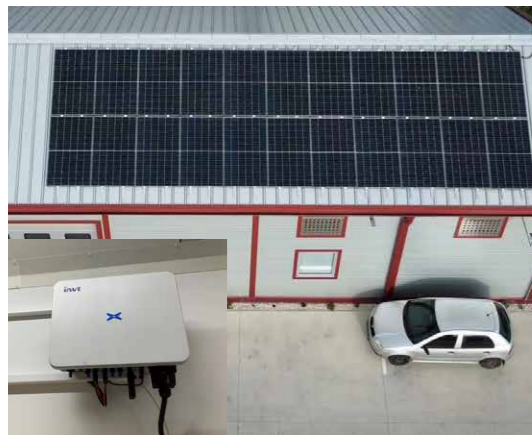
25kW Solar System in Slovakia (XG25KTR)
