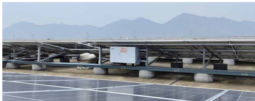
5.916MW Rooftop PV Plant in Hubei, China (XG100KTR, XG50KTR)
