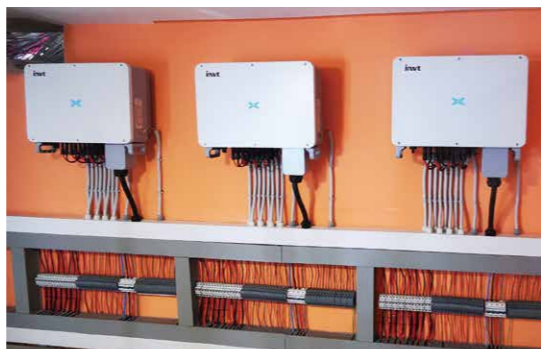
180kW Rooftop PV Plant in Lebanon (XG60KTR)
