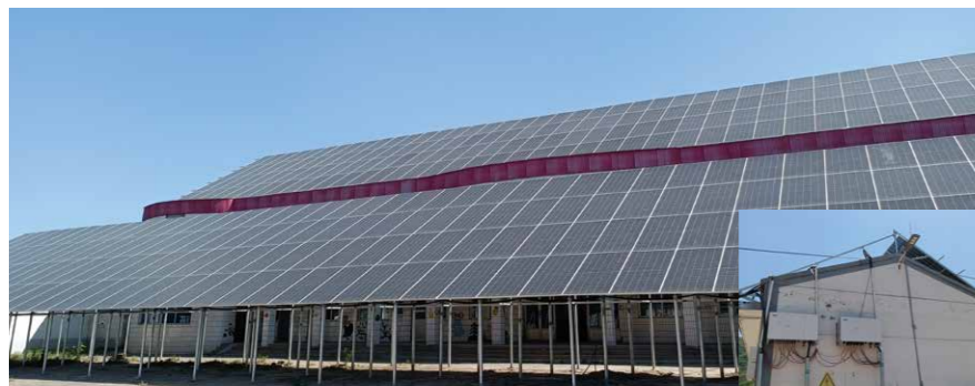
800kW Rooftop PV Plant in Shanxi, China (XG110KTR)
