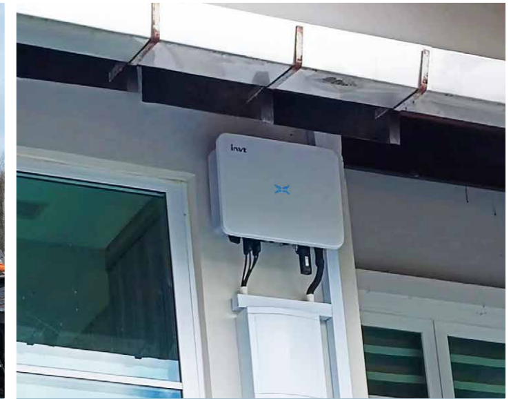
12kW Solar System in Malaysia (XG12KTR)
