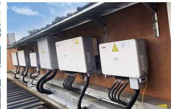
522kW Rooftop PV Plant in Zhejiang, China (XG110KTR, XG60KTR, XG50KTR)
