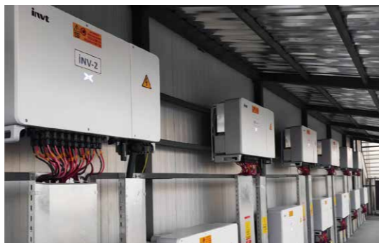
2MW Rooftop PV Plant in Türkiye (XG110KTR)
