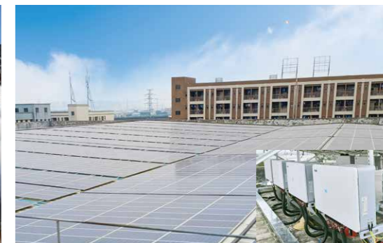
1.1MW Rooftop PV Plant in Guangdong, China (XG110KTR, XG30KTR)
