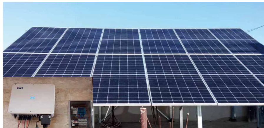
30kW Solar System in Israel (XG30KTR)
