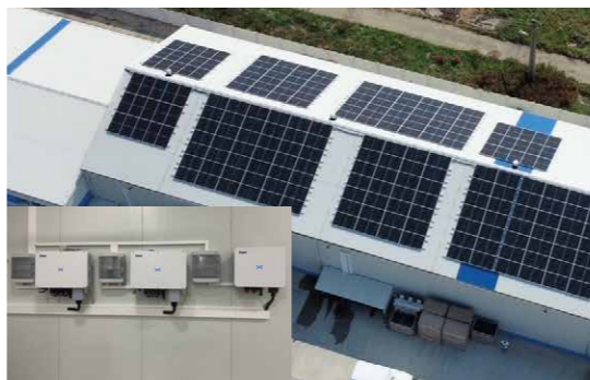
125kW Rooftop PV Plant in Slovakia (XG50KTR, XG25KTR)
