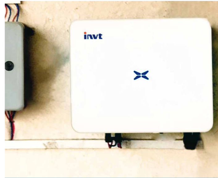
10kW Solar System in Armenia (XG10KTR)
