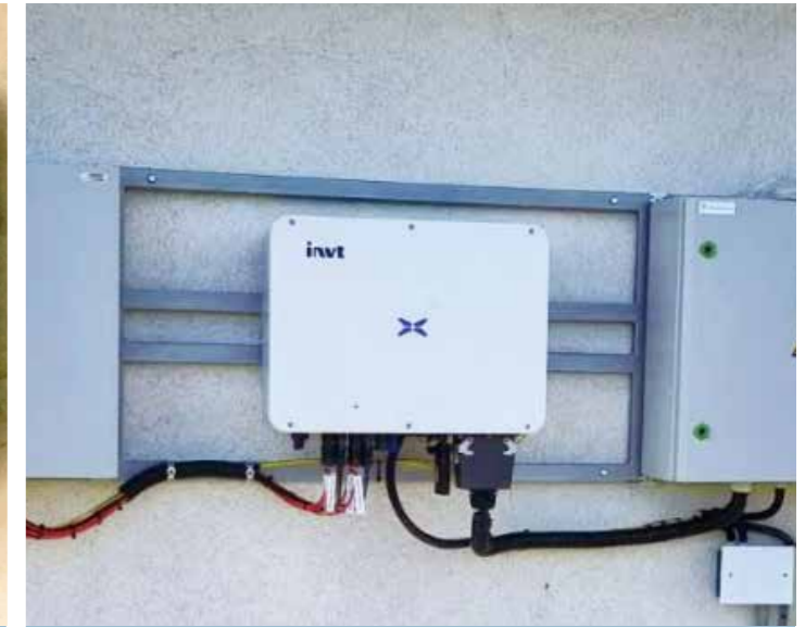
30kW Solar System in Serbia (XG30KTR)
