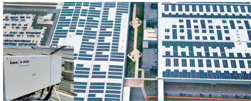
5.99MW ENOVATE Motors EV Manufacturing Base PV Plant in Changsha, China (XG110KTR, XG50KTR)
